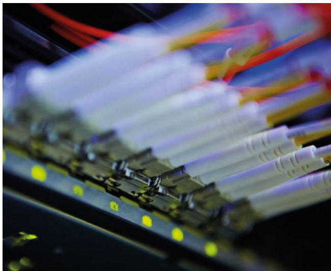
The Frankfurt data centre market remains robust and has become a key location for cloud players.
