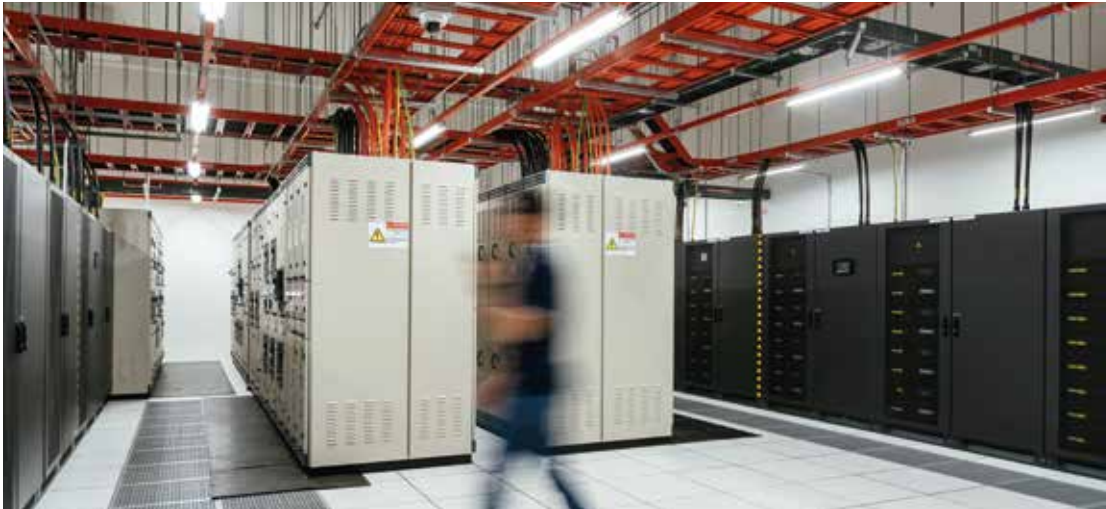
Keppel DC REIT's clients are primarily from the internet enterprises, IT services and telecommunications industries.
