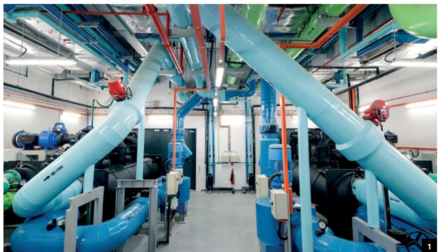
1. The report scope outlines practices in Keppel DC REIT's colocation data centre assets that the Manager has operational oversight of.
