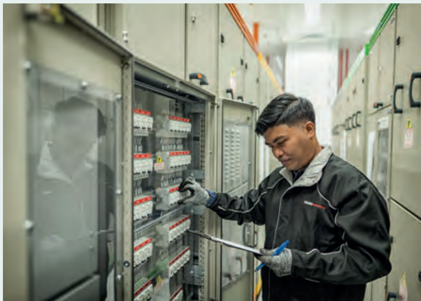
The scope of the Report covers Keppel DC REIT's colocation data centre assets, which the Manager has operational oversight of.
