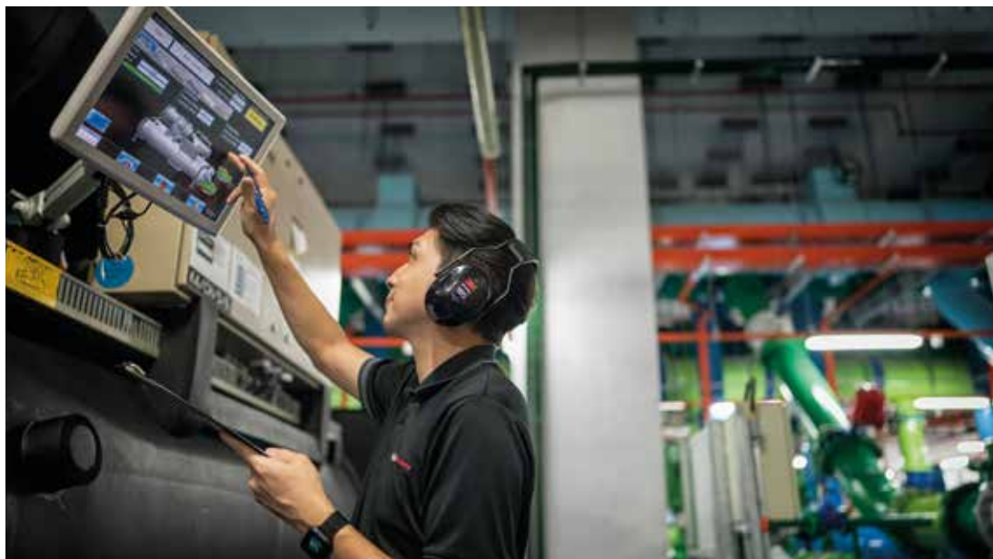
Keppel DC REIT supports climate action by adopting feasible technologies and approaches to reduce emissions and energy consumption.
